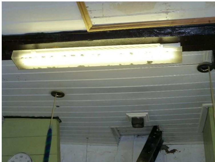
The picture above shows a typical strip light with diffuser, now with some debris building up.
